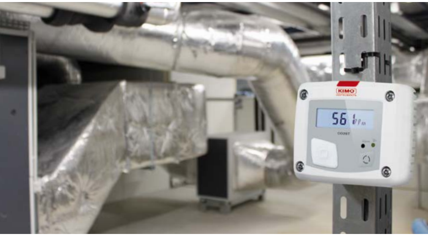
CO2ST mounted in the air handling unit of an industrial infrastructure.
