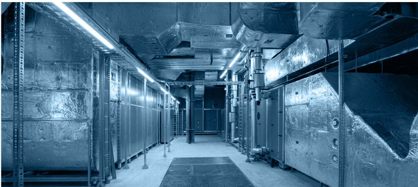
Air conditioning system of a shopping center in Zurich - ©balakate/123RF.COM
