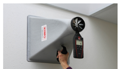
Airflow measurement using a cone with a vane probe anemometer
