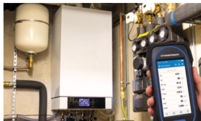
Annual domestic boiler inspection
