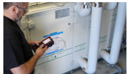
Differential pressure control on air handling units © Isatec
