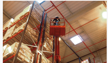
Installation of data loggers as part of biannual cartography in high-volume warehouses.
