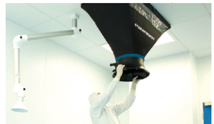
Airflow control in hospitals
